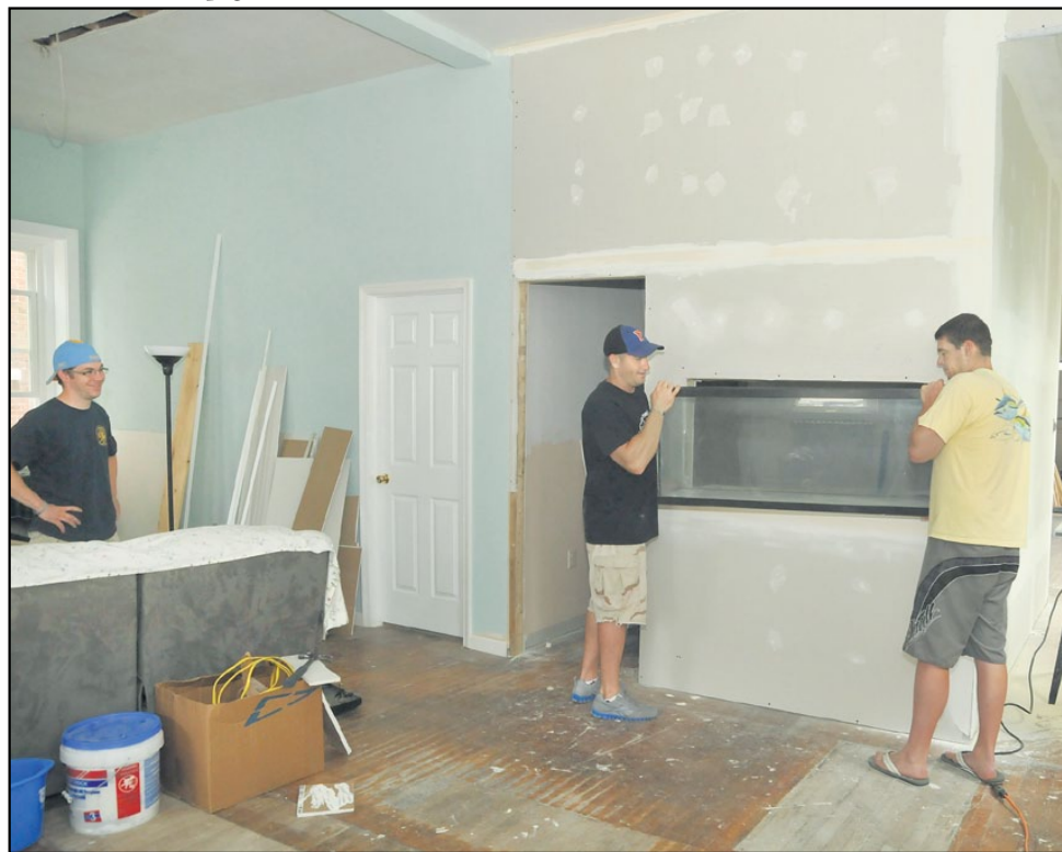
Leone and Haney position an aquarium into a wall in the dining/living room of the facility, which was once the lobby of the post office. The group, with the help of volunteers, hopes to have the renovations completed by August of this year.
